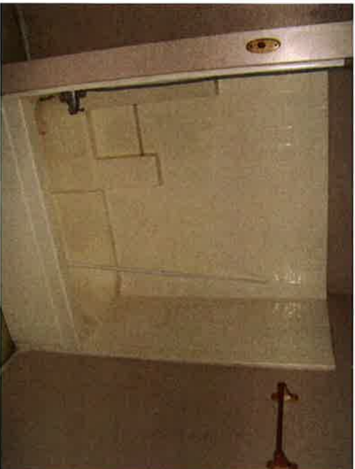
Tub/ Shower unit in bathroom
