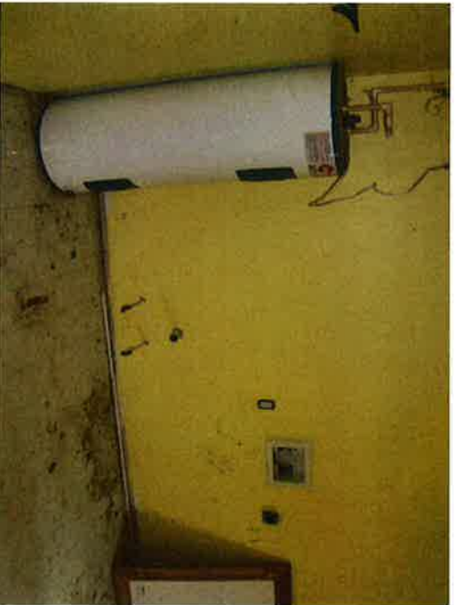
Water heater in utility
